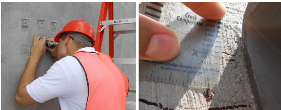
303 304 Figure 6 - Measuring crack with microscope (left) and card (right)
